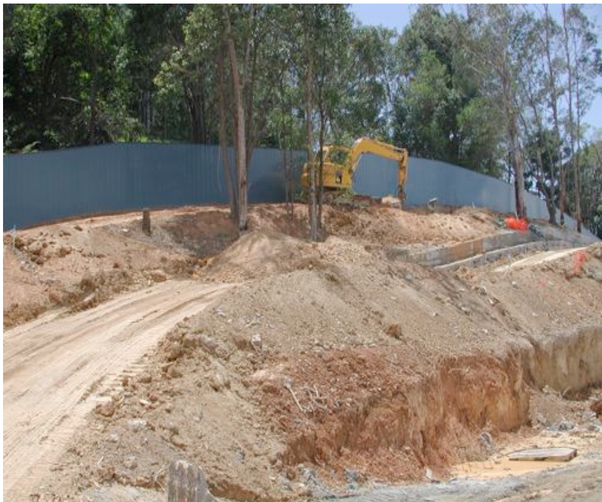
Photo 3.1 Permanent noise wall near Rajah Road being constructed early in the construction phase.
