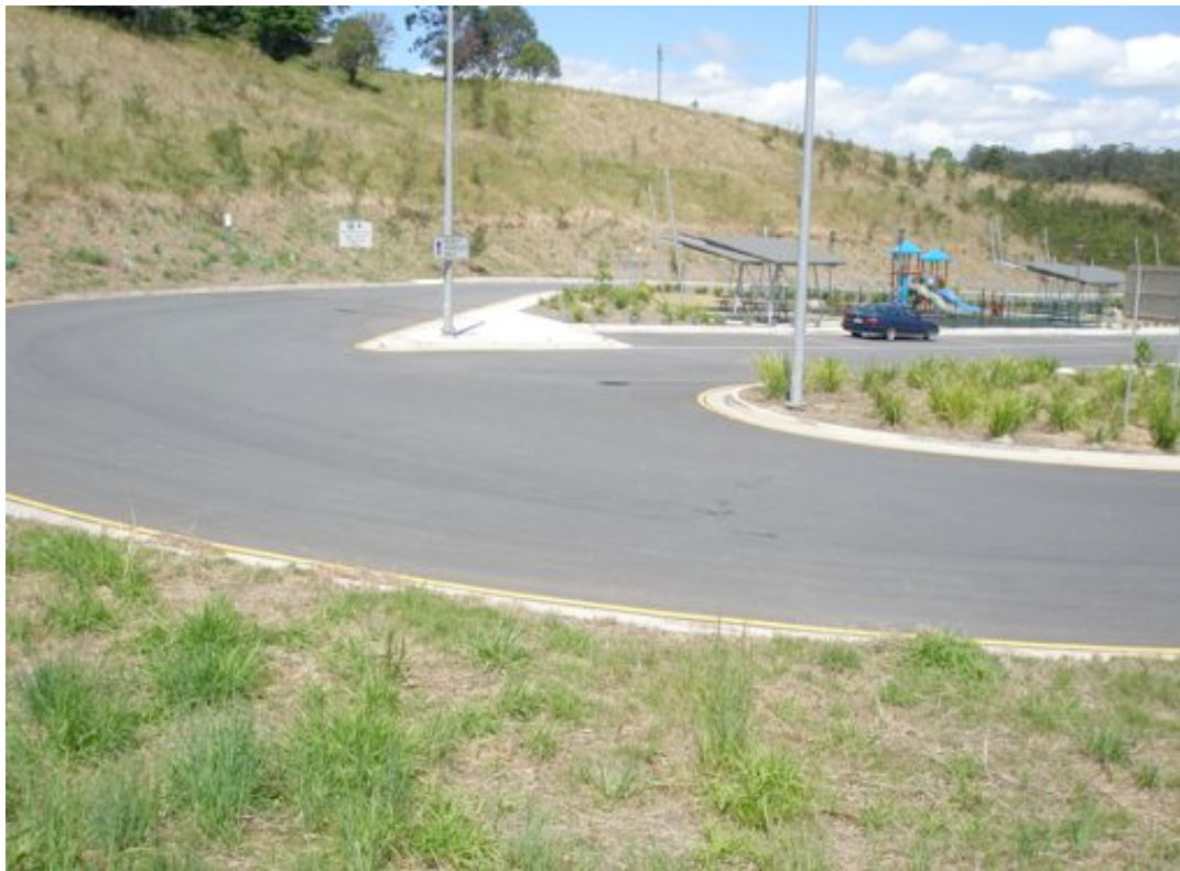
Photograph 3.34 The stabilised batters at the Yelgun Rest Area. The vegetation appears brown as a consequence of recent mowing.
