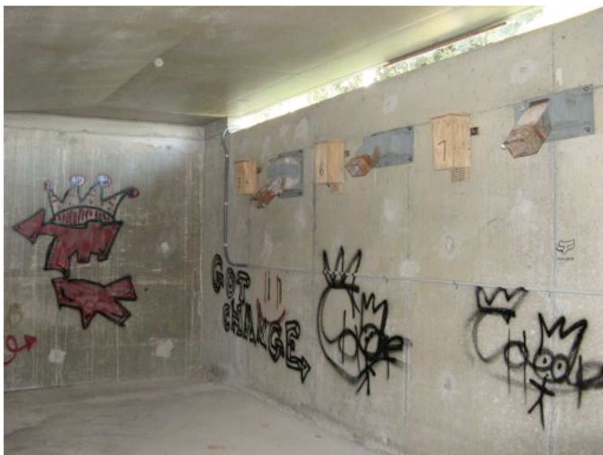
Photograph 3.32 The northern abutment of the Brunswick River Bridge showing the graffiti that has been produced by persons entering the abutment illegally. This activity may also have impacted upon the use of the boxes which are visible on the right-hand wall.
