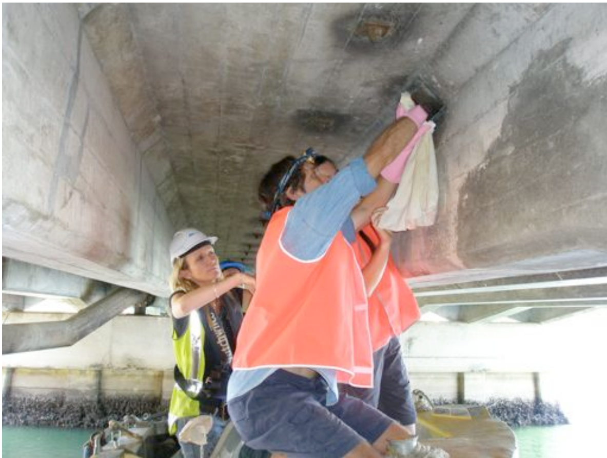
Photograph 3.28 Removal of fishing bats from scuppers in the old Brunswick River Bridge prior to demolition.
