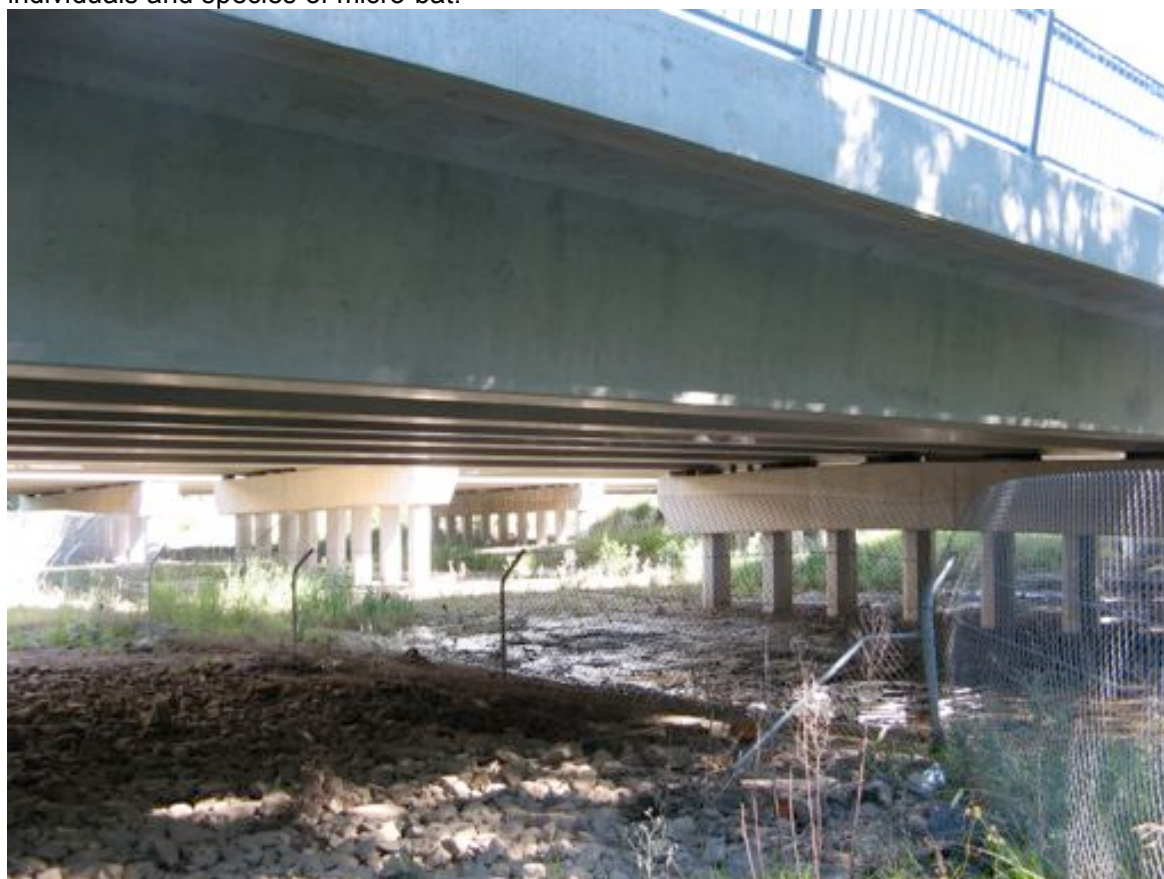
Figure 3.30 The Pacific Highway Road Bridge over Marshalls Creek, Billinudgel, local access road as viewed from the eastern edge of the southern abutment.
