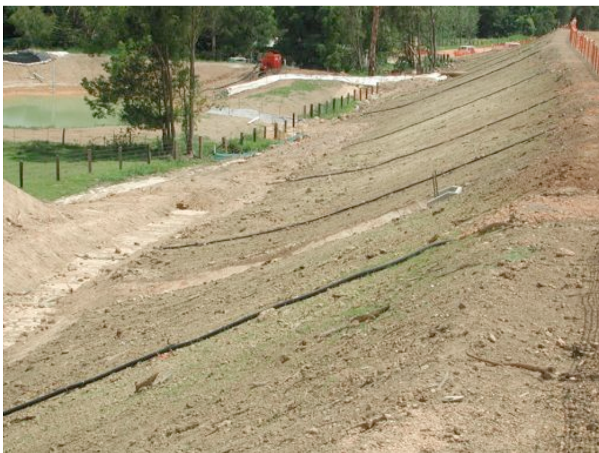
Photograph 3.21 Progressive revegetation was undertaken throughout the construction phase. This assisted with both erosion control and dust management.
